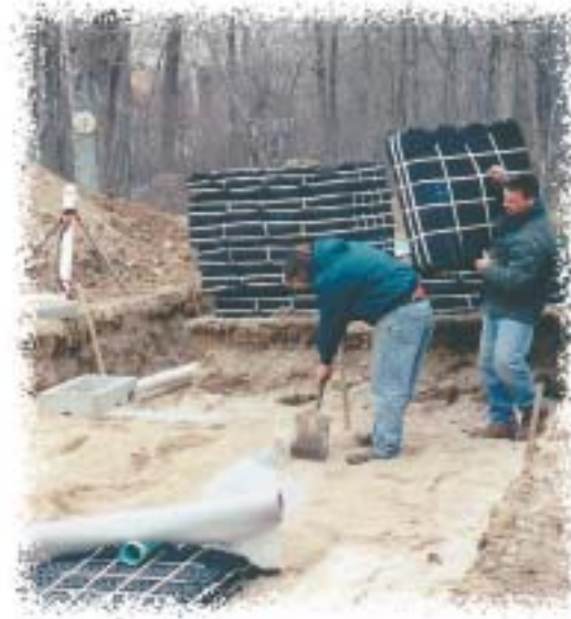
Technicians install an In-Drain system supplied by Eljen Corporation. The system includes Bio-Matt fabric that facilitates biomat growth while preserving infiltration capacity. Superior Septic designs and installs conventional septic systems and replaces and upgrades existing systems.
